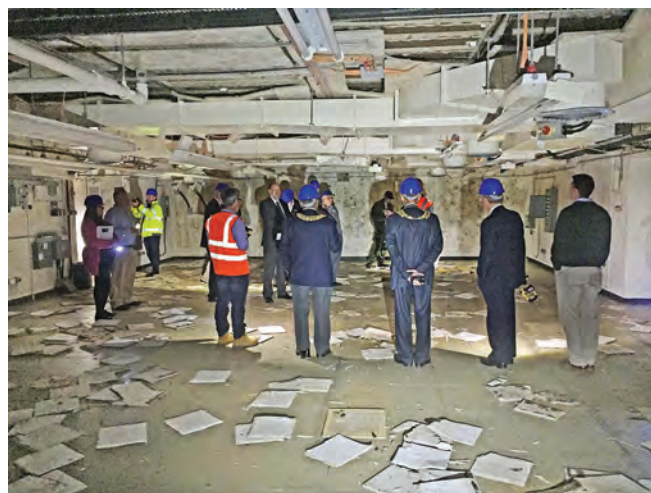
The VIP group is seen in one of the upper floor rooms damaged by condensation which caused many of the ceiling tiles to fall. Photo Rob Jacobs
